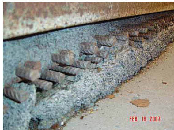
Side view of overlay showing congestion of reinforcement
