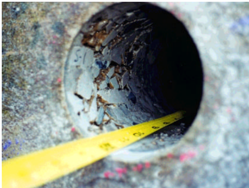
Figure 10. View inside core hole showing poor consolidation
