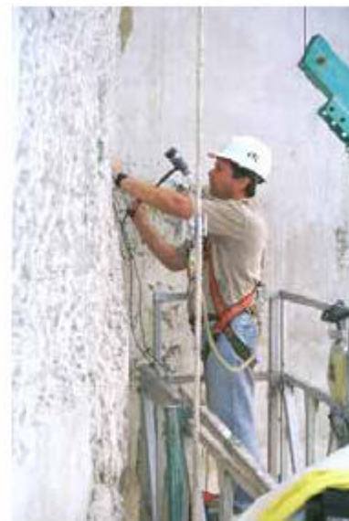
Testing for honeycombing in slip-formed silo
