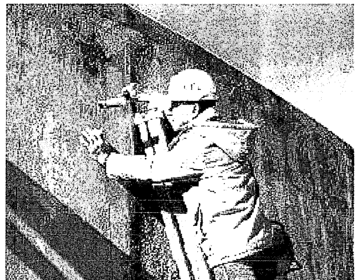
Figure 1. The s'MASH used for detection of the dynamic stiffness of a structural RC member.
