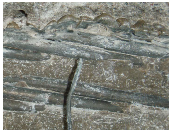
The excavated duct at location (1) reveals that some of the strands are not embedded in grout
