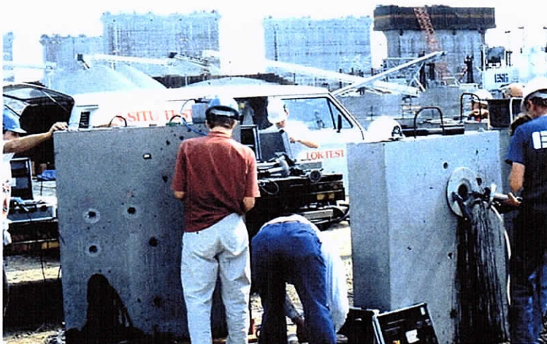
Fig.13. Training of the contractor's technicians on performing LOK-TEST and CAPO-TEST. The training course was completed with an examination and issuing of a diploma.
