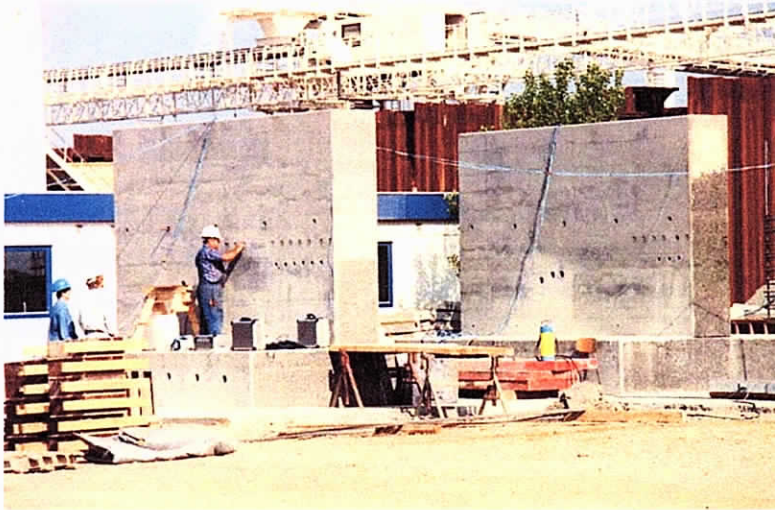
Fig.12. Trial casting, tested for chloride diffusion, strength and LOK-Test / CAPO-Test of the cover layer in relation to maturity to establish acceptable intervals.
