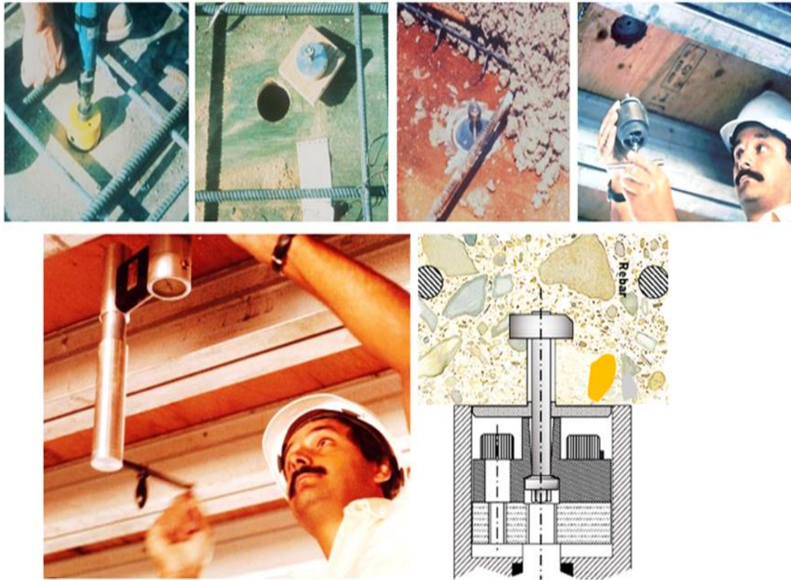
Figure 43. LOK-TEST being performed by CET Sal Fasullo, Toronto, Canada, for safe and early form stripping in a high-rise building.
