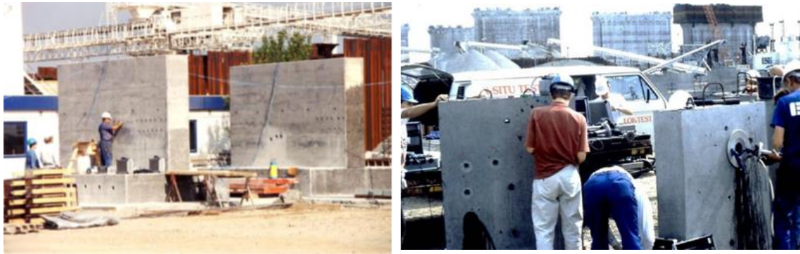
Figure 29. Trial testing for chloride migration and pullout (left) for the specified concrete, and Certification Course in testing with LOK-TEST and CAPO-TEST (right). Diploma was awarded if the technician could complete 4 LOK-TEST's and 4 CAPO-TEST's within 2 hours.
