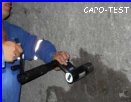
Cigar Lake Uranium Mine, Canada Strength of gunite concrete Test smart – Build right
