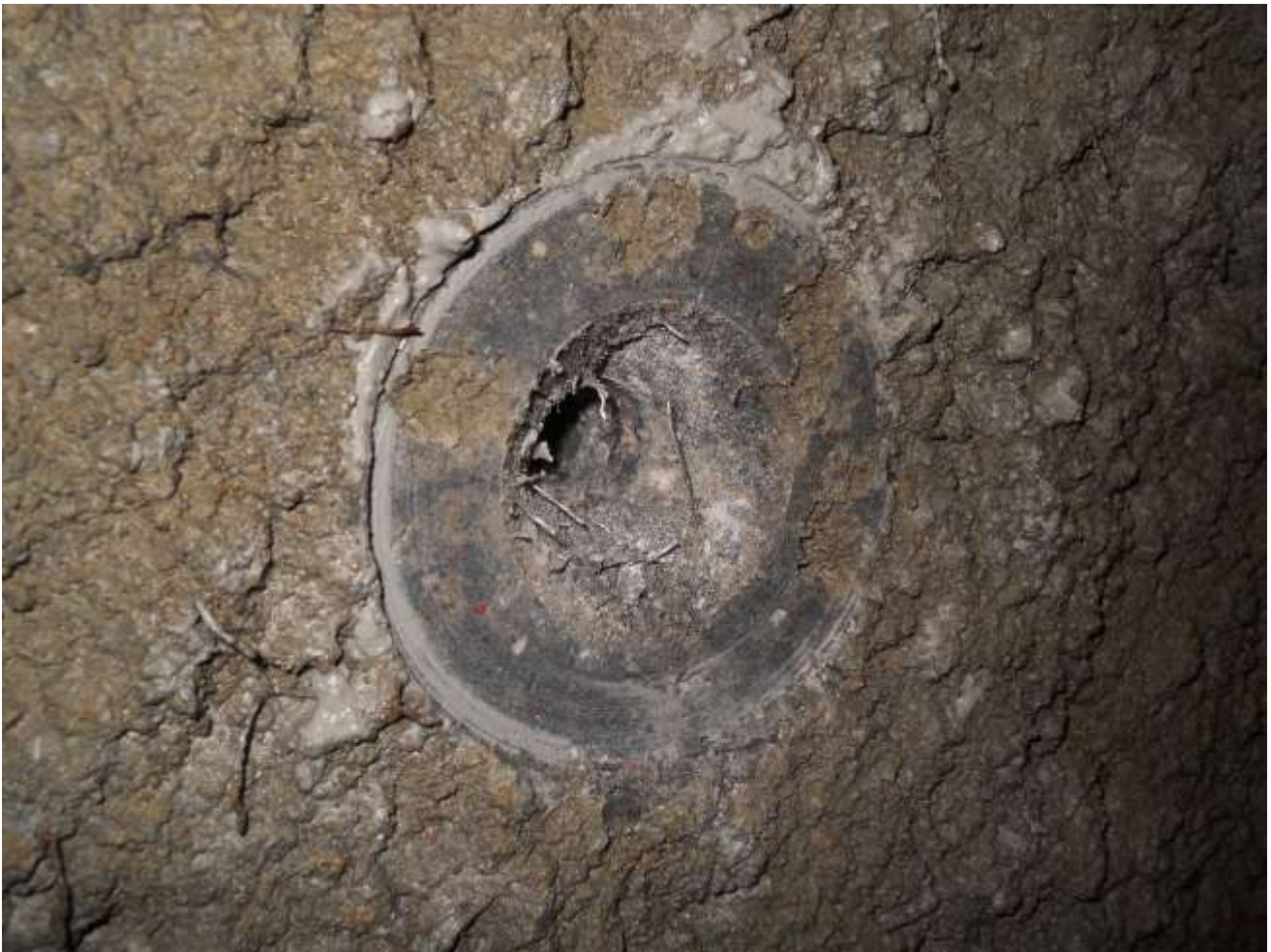
Capo-Test failure on shotcrete with steel fibers, fig. 12 Test results: 43.0 kN, 44.9 kN and 42.0 kN, shotcrete 5 weeks old
